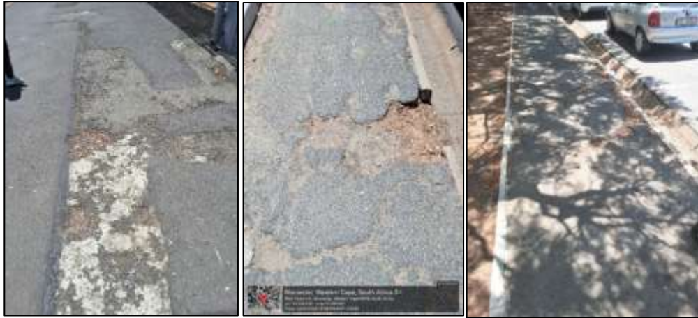
Figure 8. Damages on Sidewalks Showing (a) Peeling Off Asphalt Layer (b, c) Cracks and Broken Kerb
