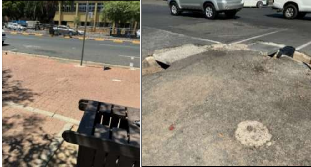
Figure 9. Paved Walkway Showing Uneven Surface (a), Pedestrian Crossing (b)
