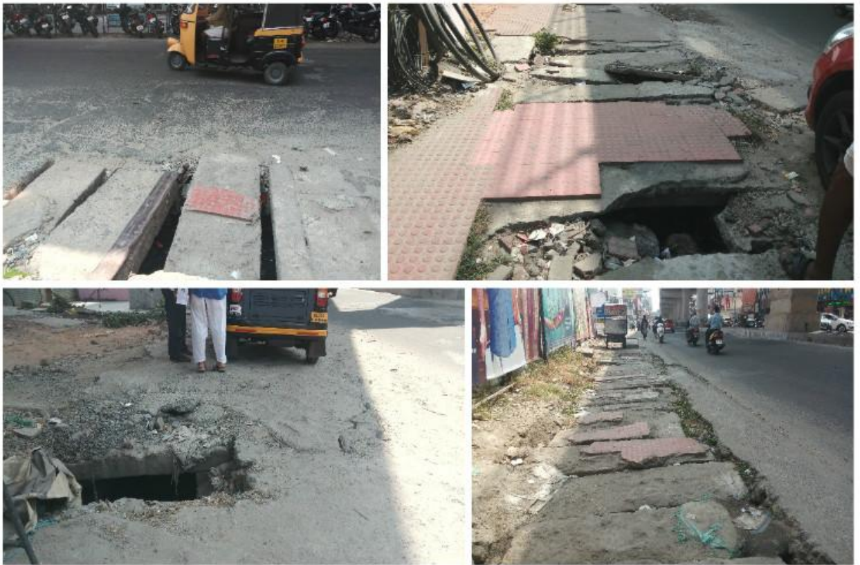
Figure 2. Broken Footpath in Study Area
