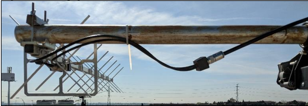
Figure 10. RF Equipment Connection to the Communication Antenna
