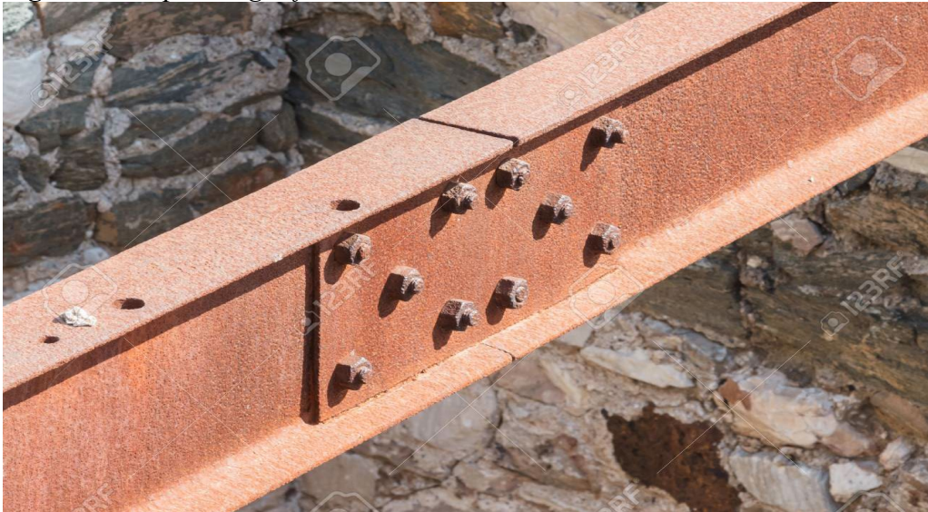
Figure 6. Sample Image of Steel Construction with Corrosion
