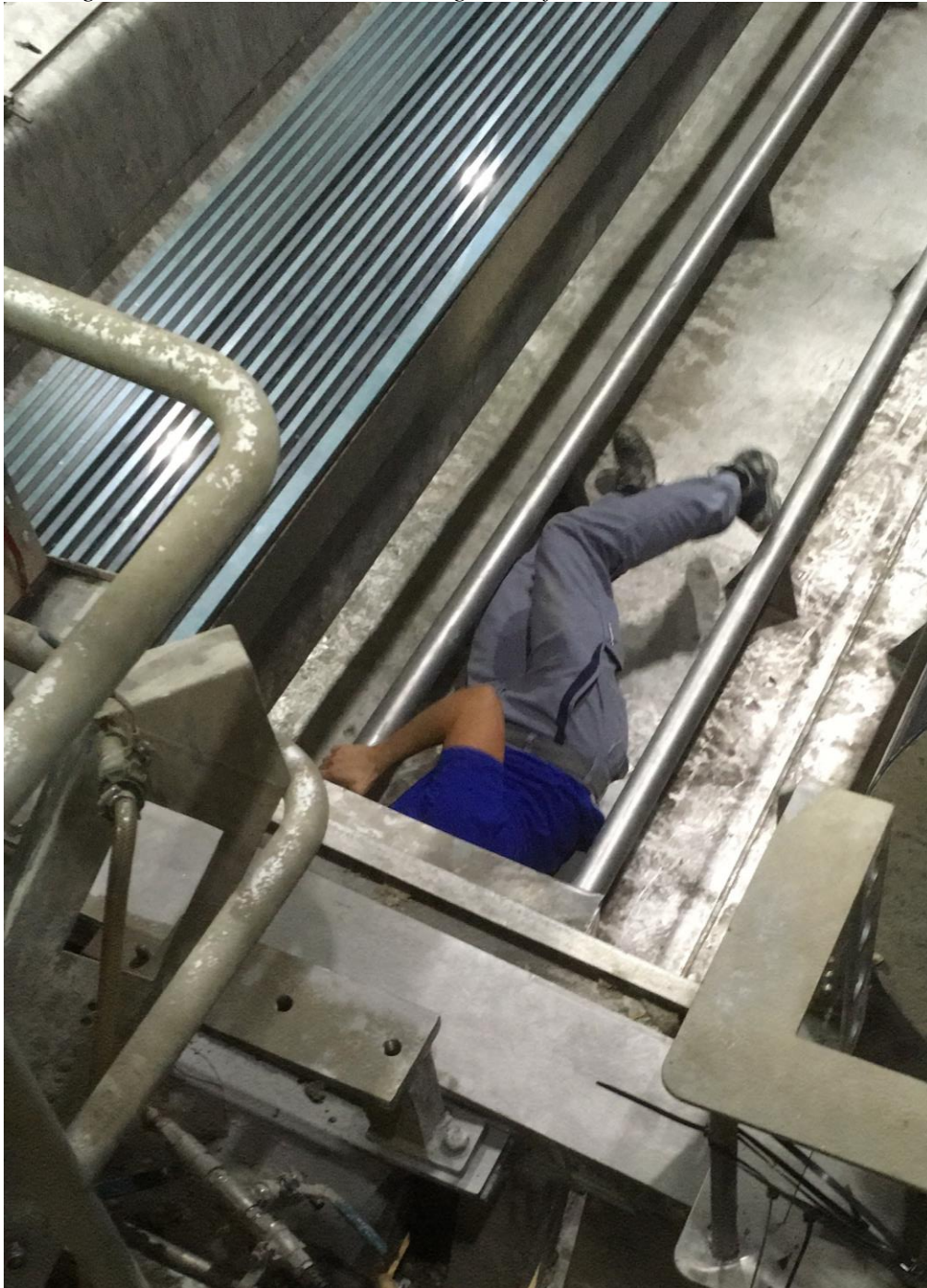
Figure 3. Suction Box. On the Left Side the Ceramic Strips (Blue) and the Slots between them (Black) can be seen. For Size Comparison in the Middle a Colleague in the Suction Box Installing One of the Sensors
