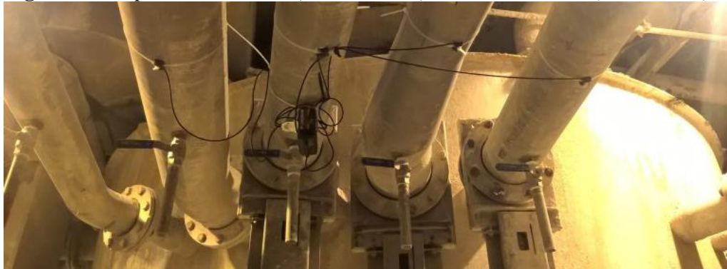
Figure 4. Temperature Sensors (Blue Arrows) and Sensor Node (Red Arrow)
