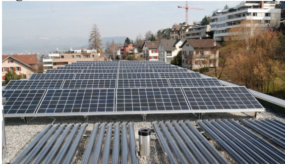
Figure 7. PV Panels Were Added on the Top Roof in the Rehabilitation Process
