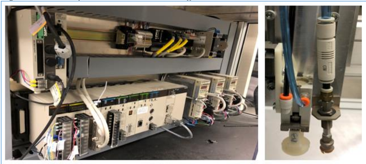
Figure 3. XYZ Gantry Robot PLC Rack and End Effectors
