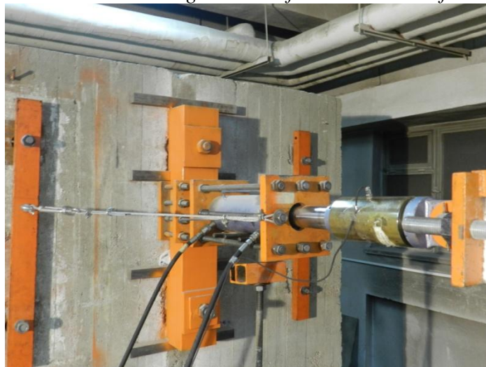
Figure 3. Steel Cables Preventing the Out-of-Plane Motion of the Jack
