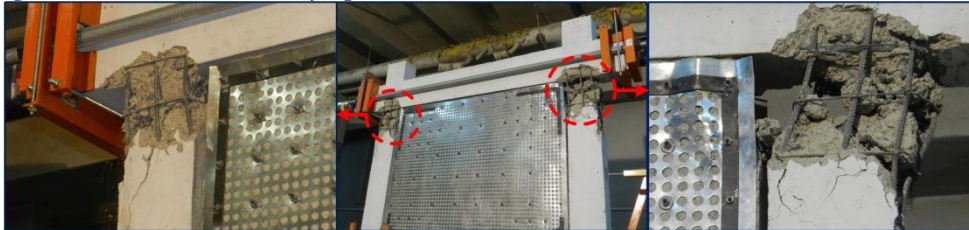
Figure 8. Failure Mode of Specimen S1ZN200
