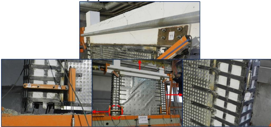
Figure 11. Failure Mode of Specimen S1ZY150
