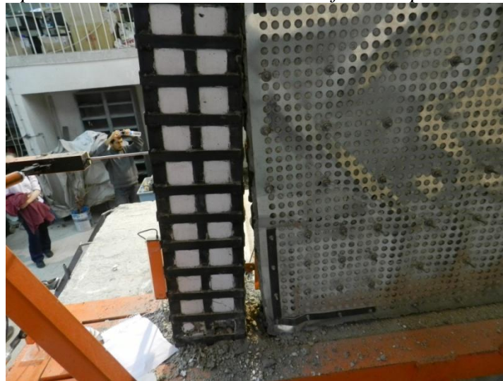
Figure 21. Separation at the Wall-Column Interface in Specimen S1ZN150
