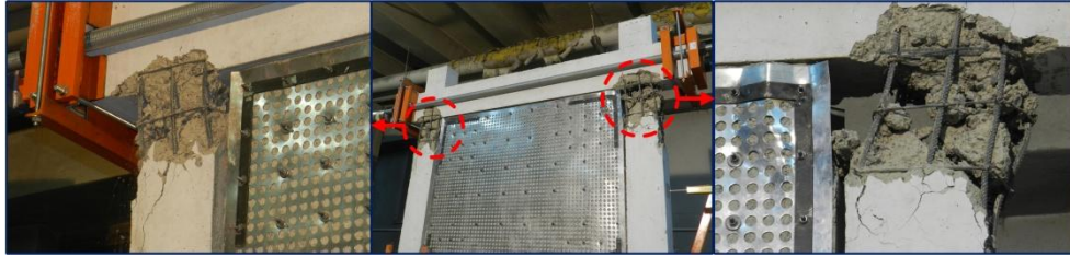
Figure 2. Shear Failure of the Columns in Specimen S1ZN200
