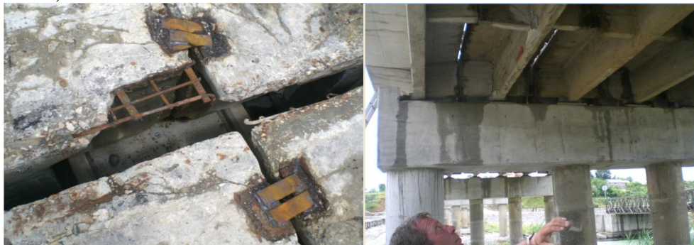
Picture 5. Photos of Deteriorated Concrete and Reinforcement. (Damage Details)
