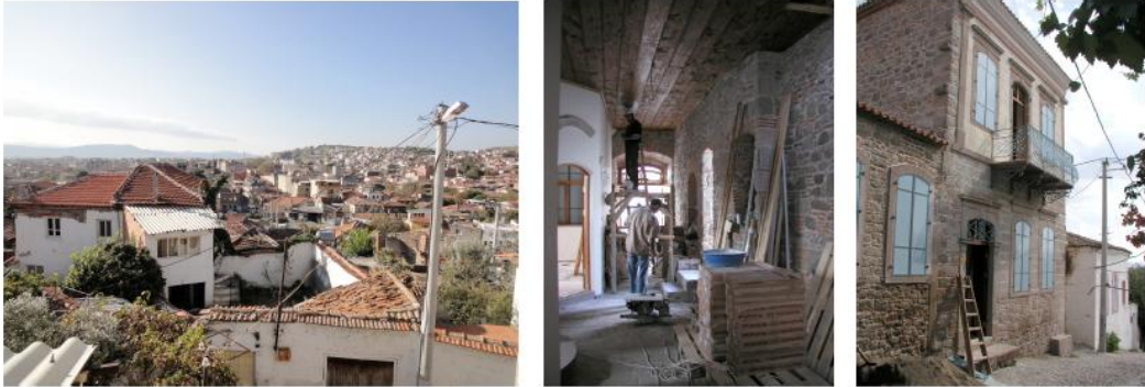
Figure 13. Various Traditional Dwellings Show the Richness of Living Culture and Art in Bergama/ Reconstruction of Old Building or Traditional House into Guesthouses, Coffee Shop or Restaurant will be a Way to Solve Problems of Conservation and Local Economy/ Credits: Authors
