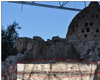
Figure 20. Collapsed Dome and Reconstructed Wall, İsmail Bey Bath, İznik
