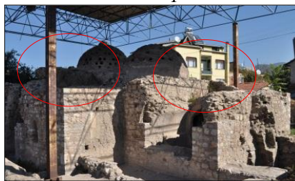
Figure 11. İsmail Bey Bath and its Collapsed Parts, İznik
