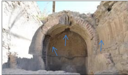
Figure 21. Cracks Under the Vault
