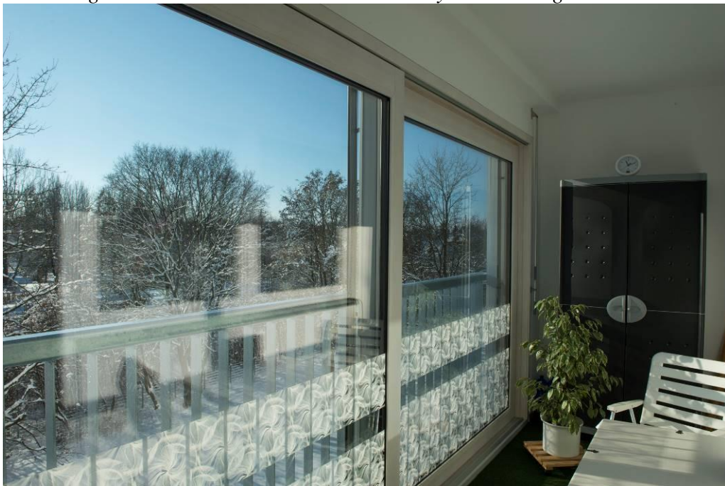
Figure 10. Project Grüntenstraße, Augsburg. The Existing Balconies were Converted into Winter Gardens thus Generating More Living Space and Increasing Sound iIsulation Towards the Nearby Street. Image Frank Lattke
