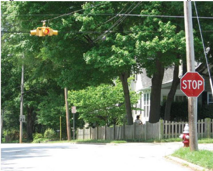
Figure 1. Intersection Standard Overhead Flashing Beacon
