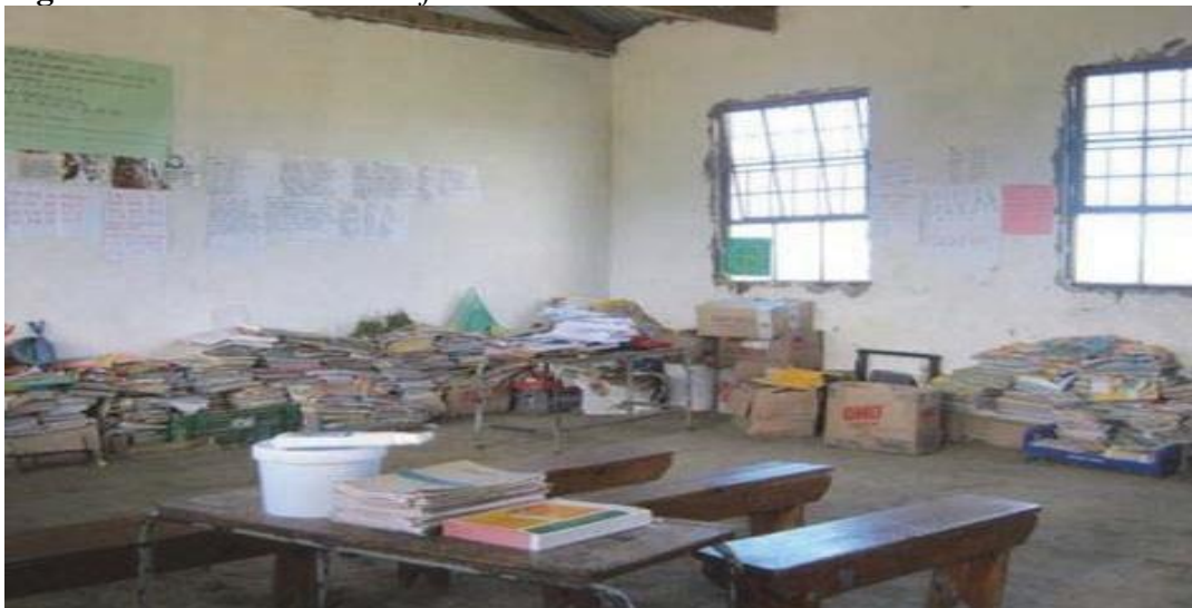
Figure 2. Poor Classroom Infrastructure
