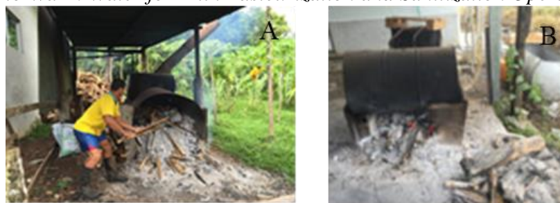
Figure 2. Wood Boilers Used in LLAFRAK (A) and San Bosco (B) Dairy Factories to Warm Water for Milk Pasteurization and Sanitization Operations
